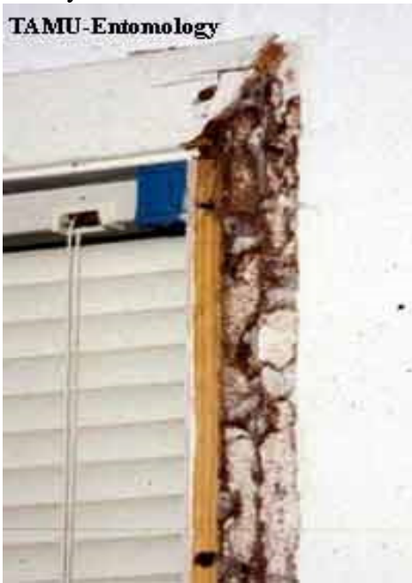
Photo of termite damage. Photo by Center for Urban and Structural Entomology, Texas A&M University.
